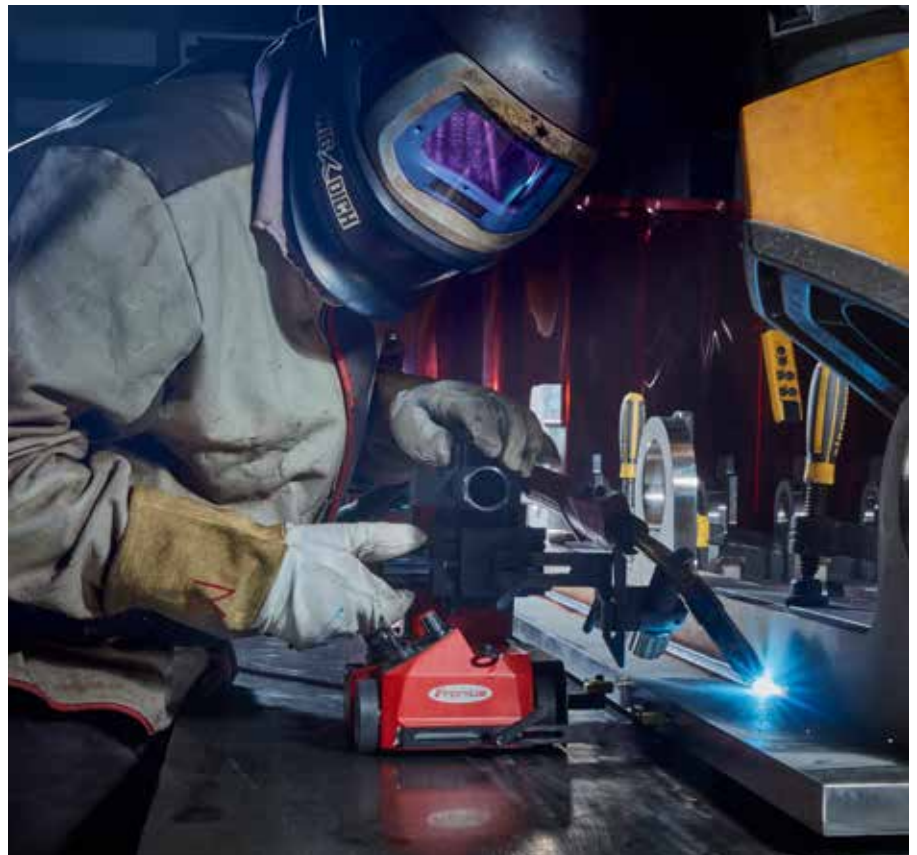
Our welding specialists are aided by a battery-powered undercarriage when applying straight welds.
